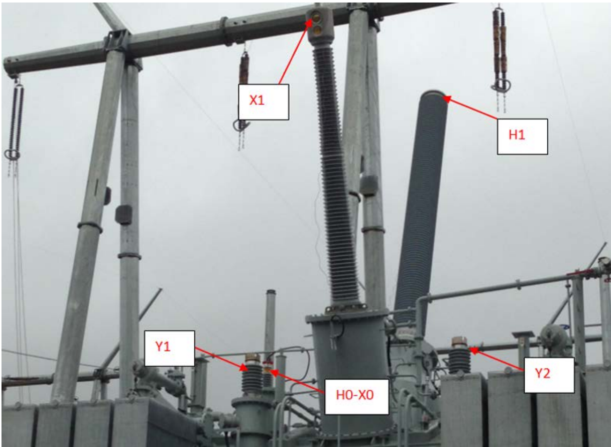
Figure 13: Picture showing the location of each bushing on single phase auto transformer with tertiary
